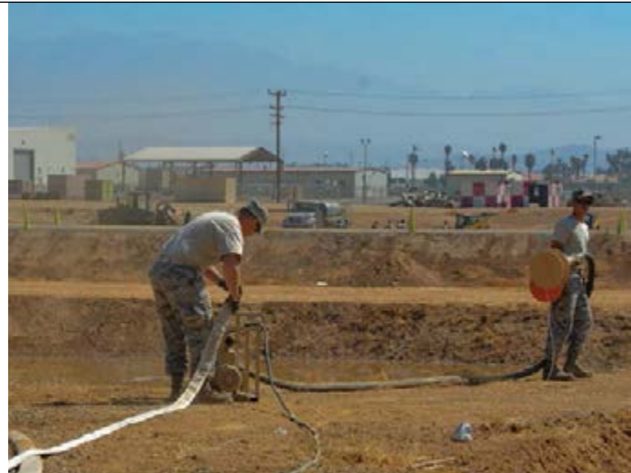
Members of the 172d Airlift Wing’s Civil Engineering Squadron prepare to drain water from a pond to process it through the Reverse Osmosis Water Purification Unit. (Photo by Tech Sgt Marsha Williams, U.S. Air Force)
