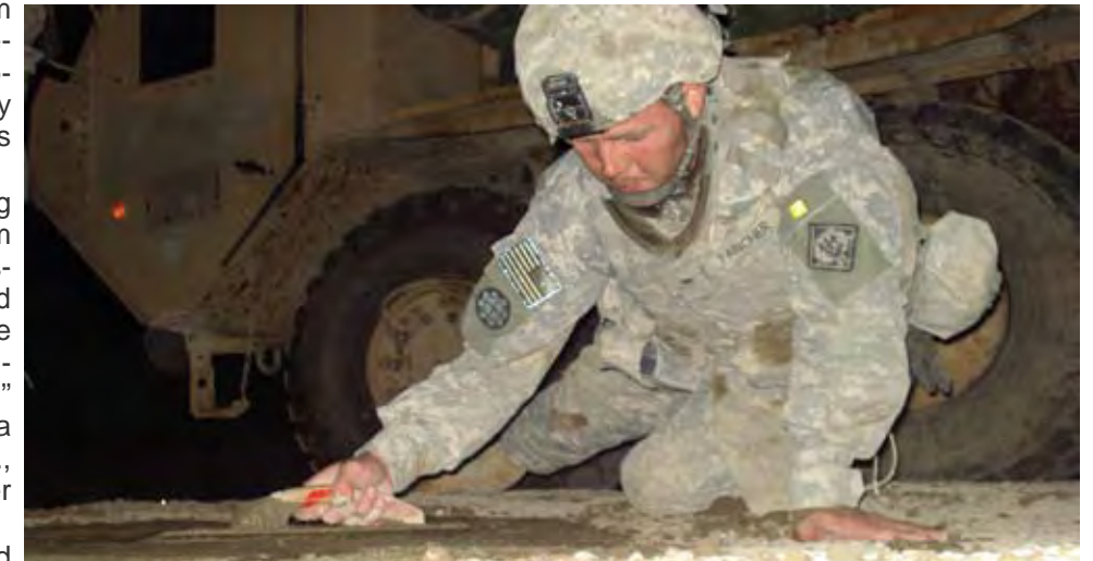
Spc. Robert Fancher, from Grenada, Miss., uses a hand trowel to smooth out concrete for rapid roadway repair in northwestern Baghdad. He is a member of the 230th Concrete Team, Mississippi Army National Guard.
