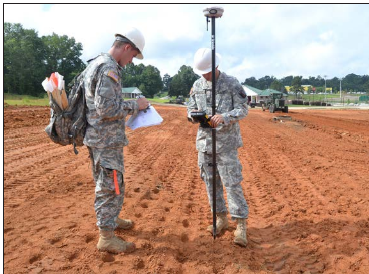
Sgt. Justin Grider and Spc. James Horn, both assigned to the 168th Engineer Brigade in Vicksburg, Miss., survey an area where a 54,000 square foot parking lot will be constructed at the Robert E. Russell Sports Complex in Petal, Miss. Mississippi Army National Guard engineering units are providing construction assistance for the city during annual training.
