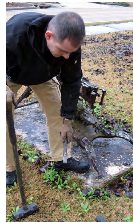
Stephen Magee, museum assistant, works to remove a MG08 Maxim Machinegun from the concrete slab housing the weapon since it was emplaced in 1938. (Courtesy photo)
